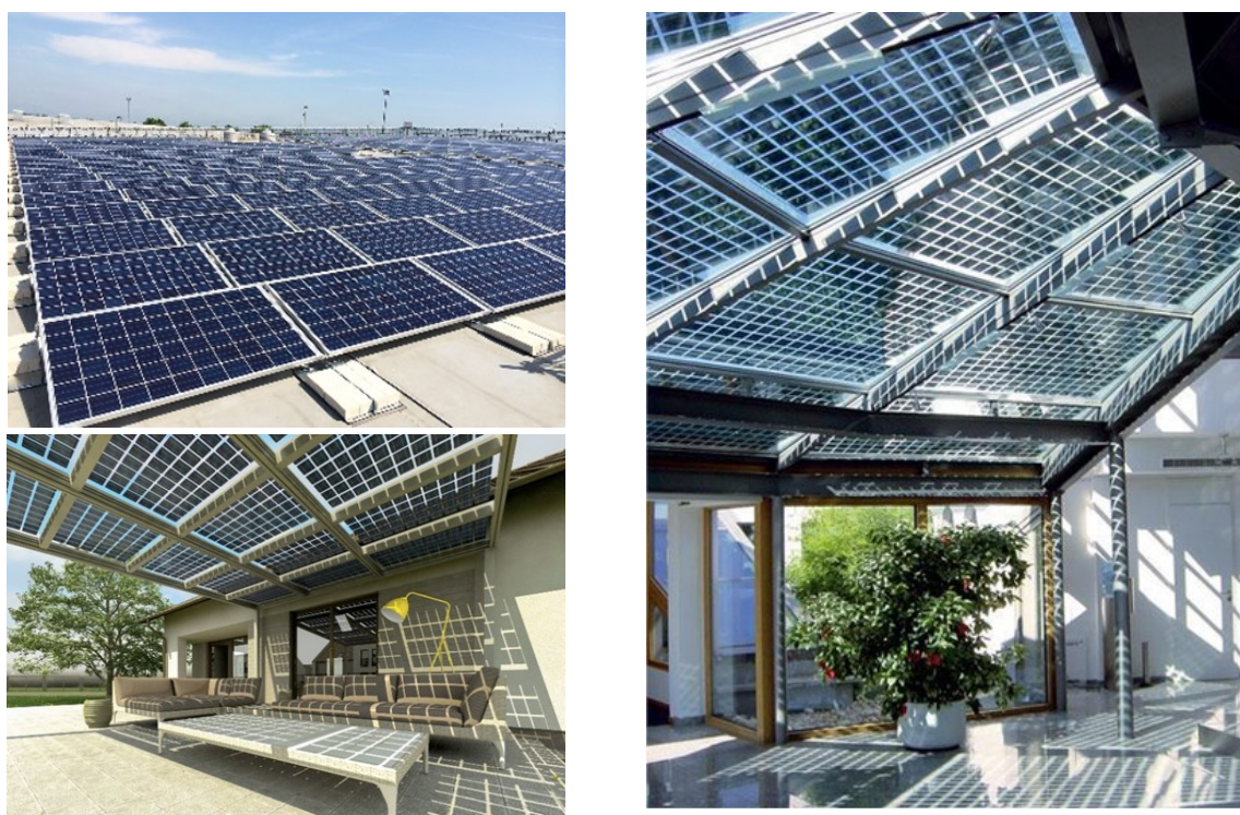
Figure 7 – Examples of PV installations
